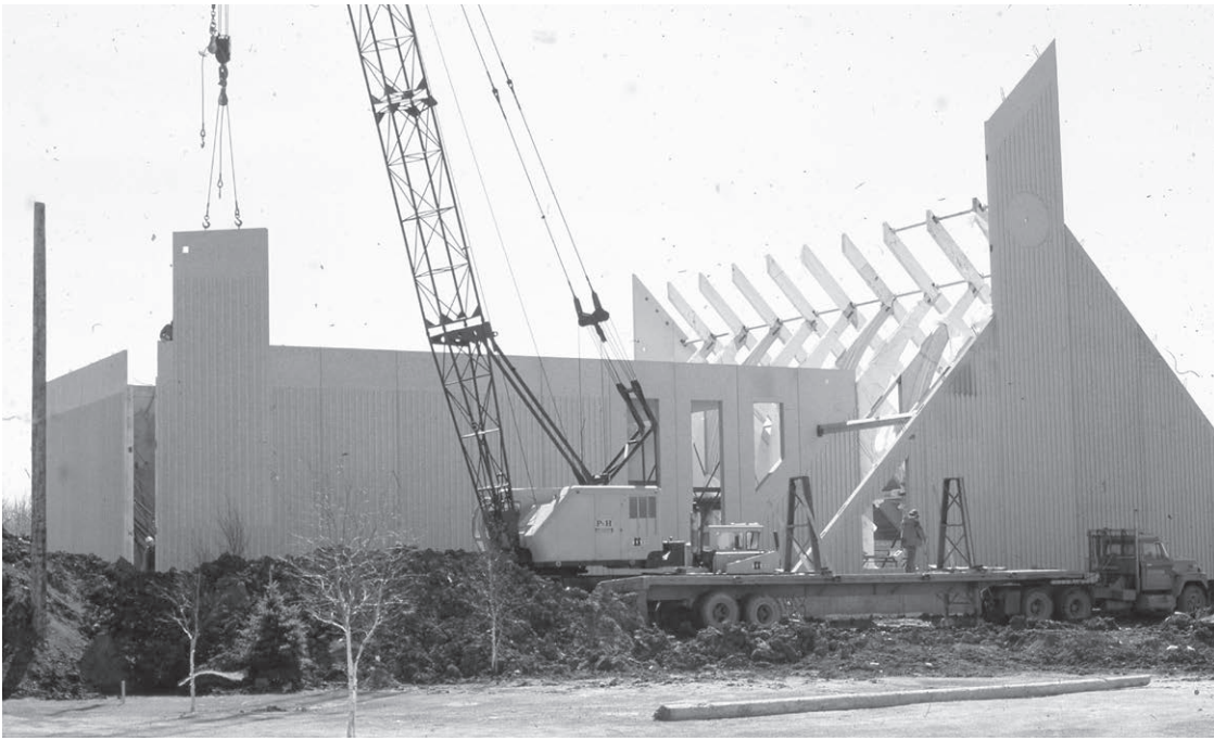
Mennonite Heritage Archives building in Winnipeg under construction in 1978. Photo credit: MHA.
