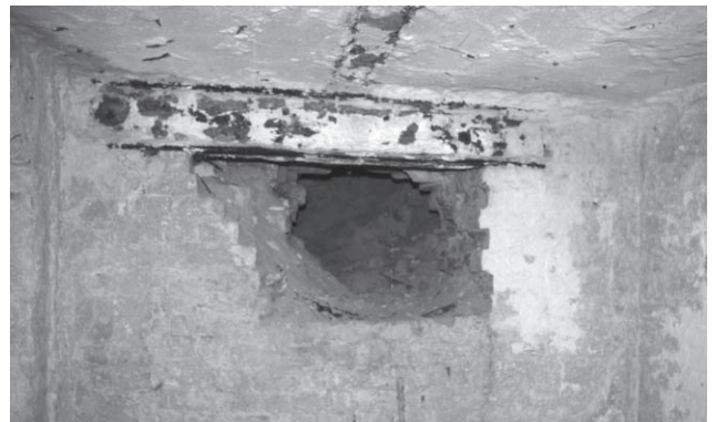
Tunnel entrance in the basement of the old Credit Union building, showing an opening in the bricked-over section.
